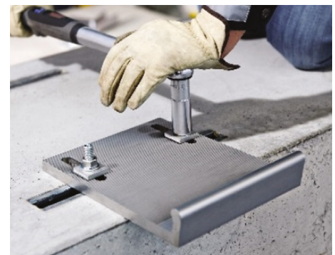
Wrong installation torque
