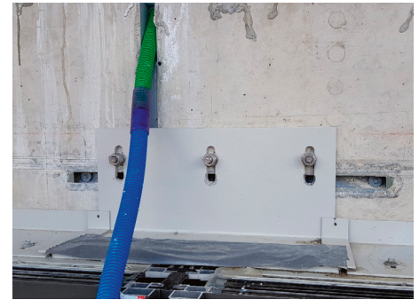
Figure 23: Use of post-installed anchors due to wrong positioning of the anchor channel
