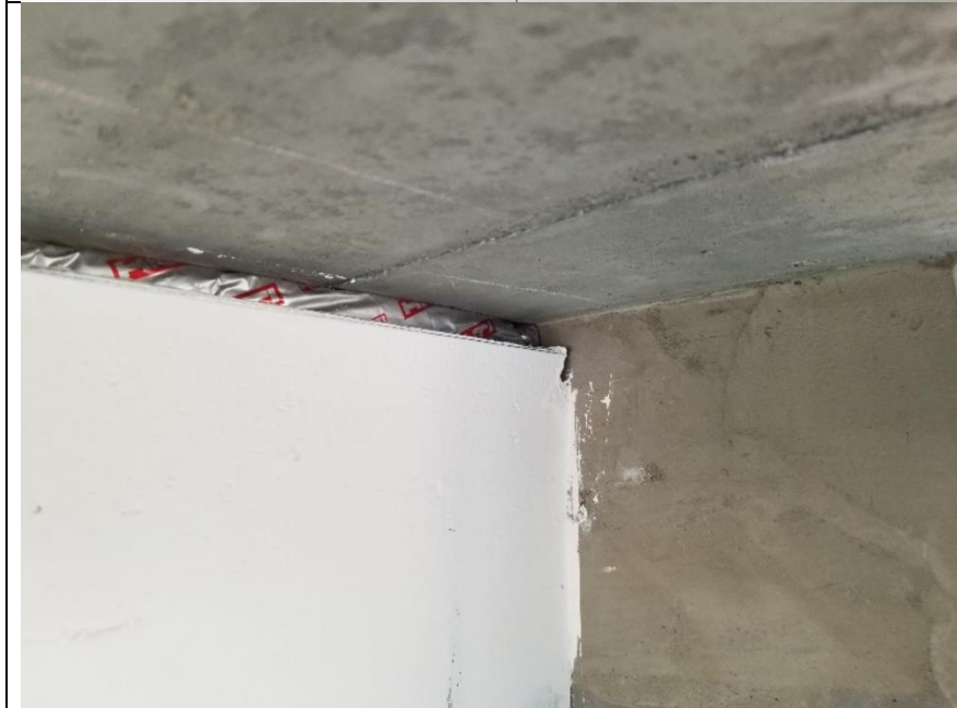
Top of wall showing Hilti CFS-TTS at top of wall
