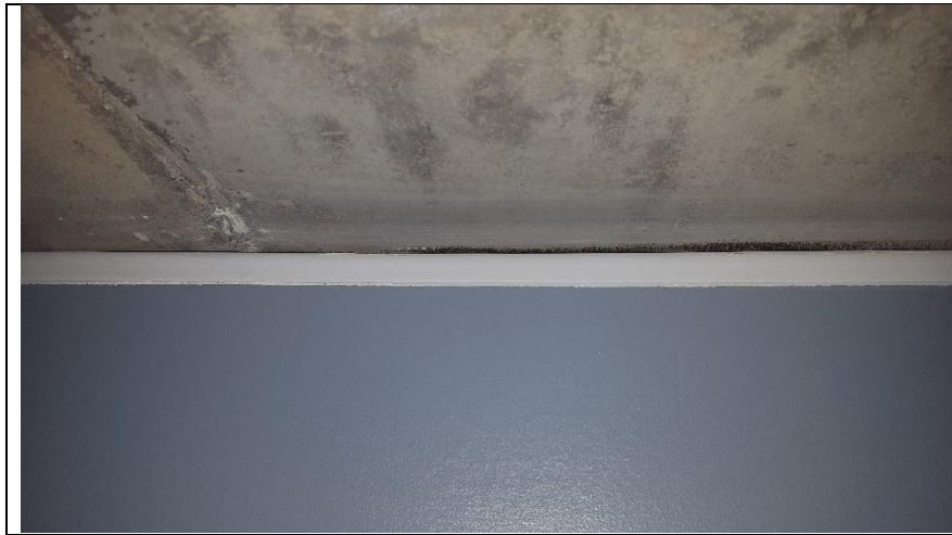
Top of wall showing variation in slab flatness and incidental gaps
