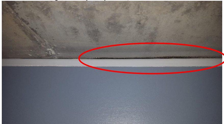
Figure 4 – Gap at top of wall, Guestroom 611
