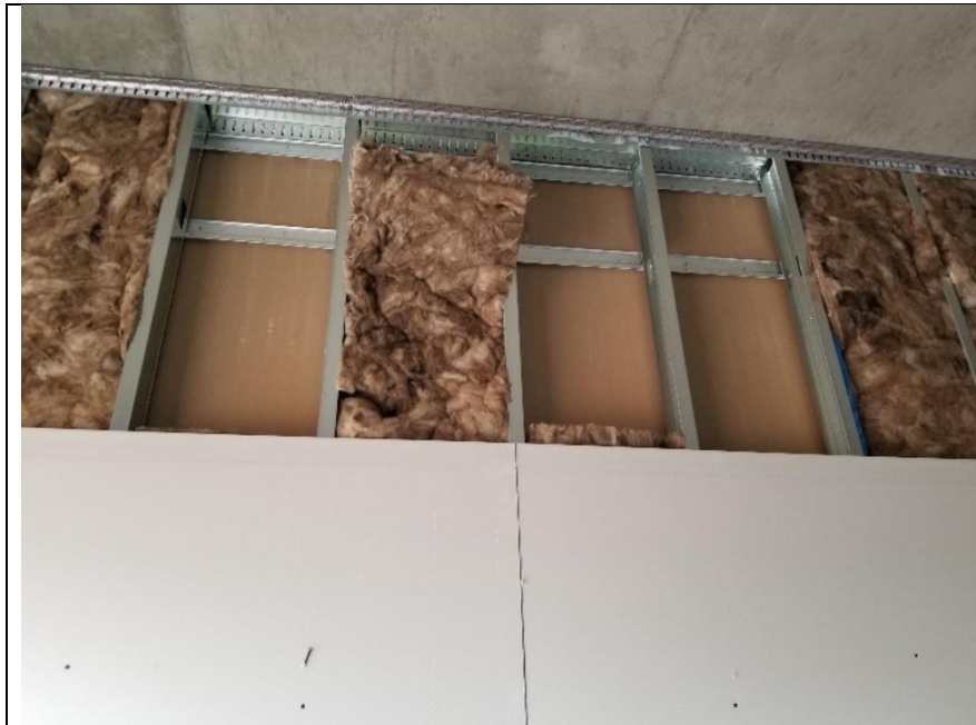
Construction of demising wall in progress showing insulation, resilient channels, Hilti CFS-TTS, and gypsum board
