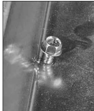
Fastener stand-off - Torque setting is too low. Increase setting by one and drive another fastener
