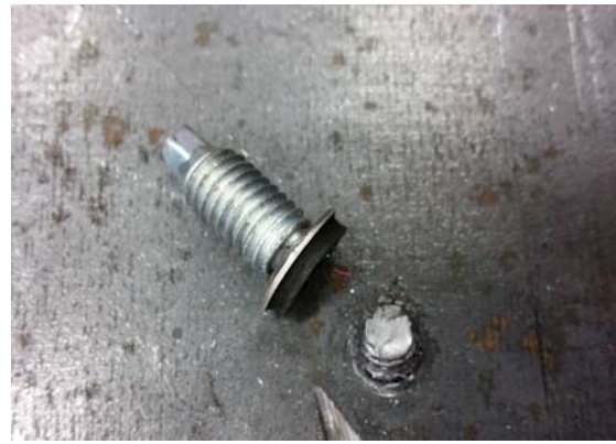
Figure 6: Typical Seismic Shear Failure – Fastener Shear Fracture
