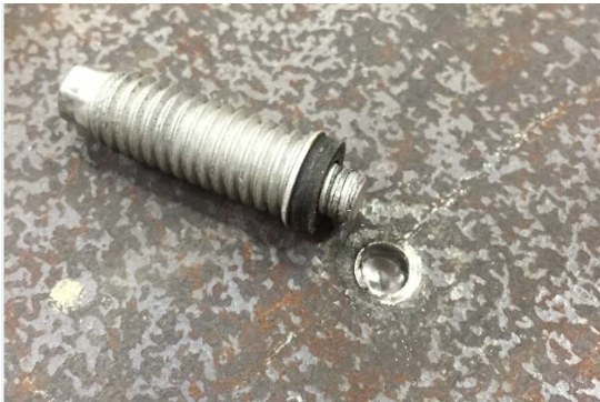
Figure 7 - Typical Tension Pullout Failure
