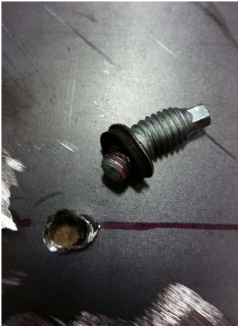
Figure 7: Typical Seismic Shear Failure – Fastener Shear Pull-out
